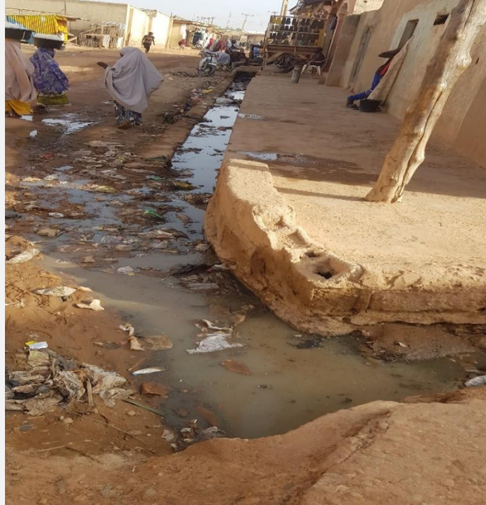
Figure 5. An Existing Drainage Alongside the Major Road showing the condition of the drainage in Tudun Yan-Lihidda Settlement, 2022
