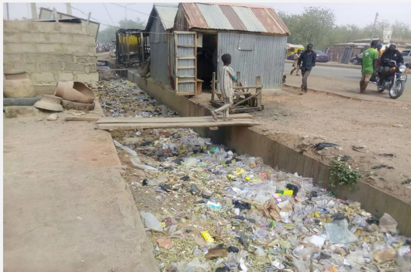
Figure 3. Waste Materials dumped inside a storm drainage in front of Kofar Guga Motor Park.
