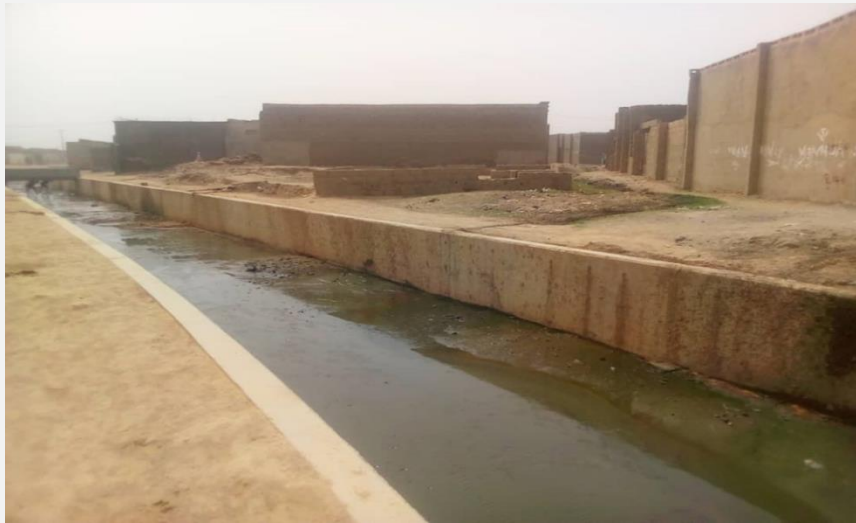
Figure 5. A section of the river converted to storm water drainage for flood control constructed by Katsina State Government from 2020 – 2021.
